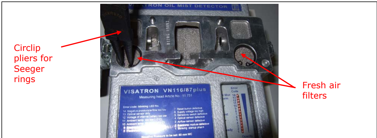
Figure 46: Exchange of the air filters
